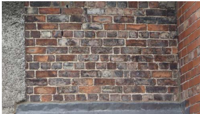
Brickwork found both at the station and the farm buildings. Technically it is called English Garden Wall Bond, a weakly bonded wall as only one course in four bonded with the inner wall.
